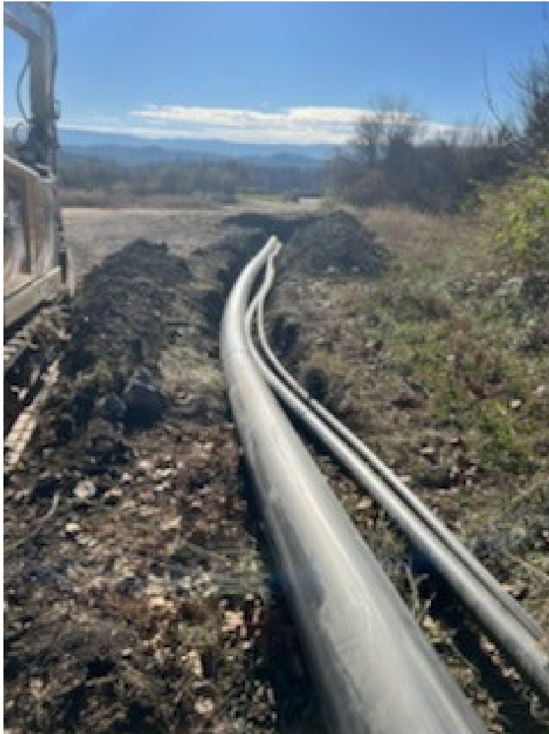
Figure 2. Installation of 12-inch Header, 2-Inch Airline, and 4-Inch Forcemain in Common Trench
