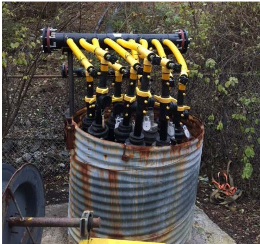
Figure 1. South Leachate Cleanout Manifold and Cleanout Tie-ins to the GCCS
