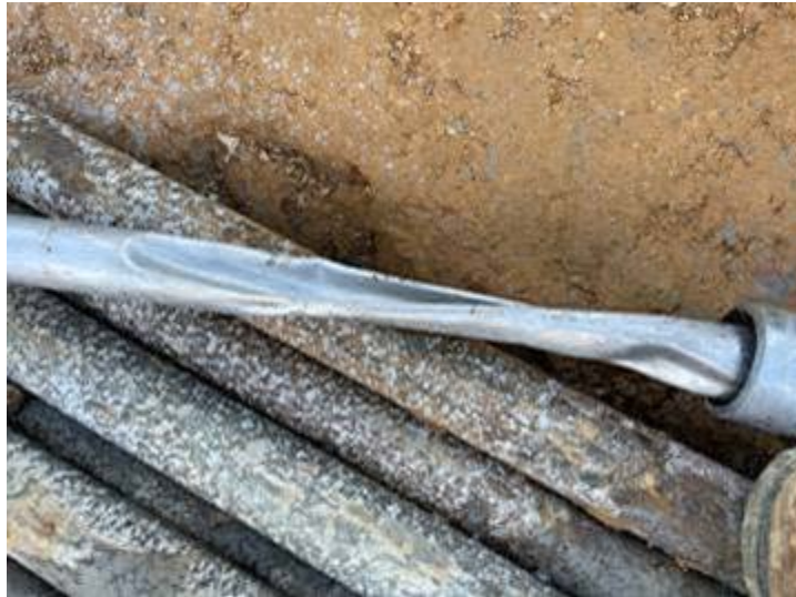
Figure 10. TP-1 Casing Damage
