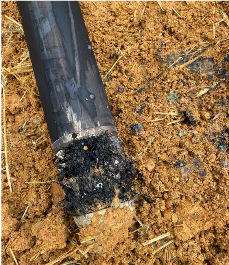
Figure 11. Material Clogging Landfill Gas Well Dewatering Pump
