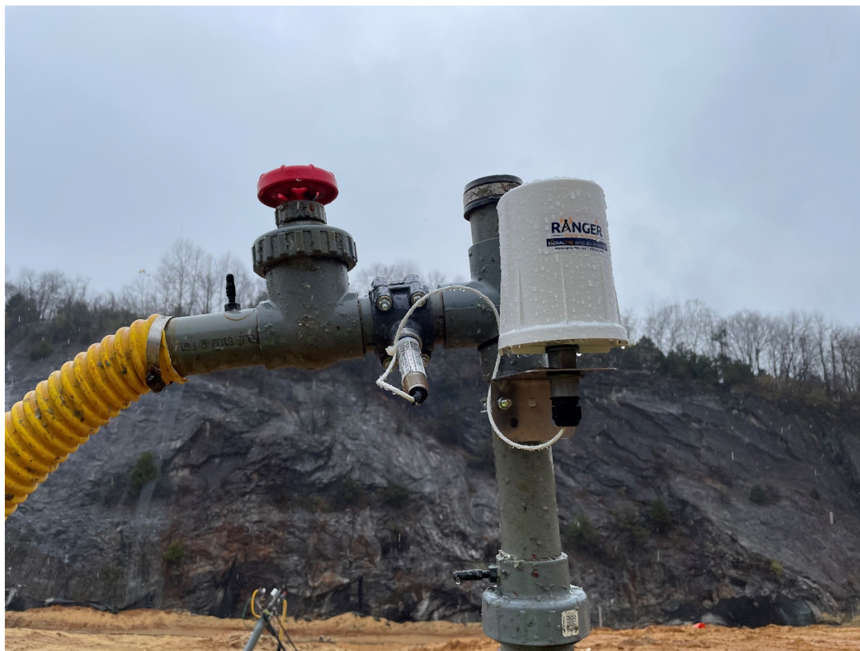
Figure 4. Wellhead Temperature Sensor after Installation
