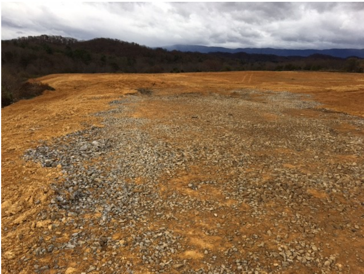
Figure 1. Intermediate Cover Placed on the Solid Waste Permit #498 Landfill
