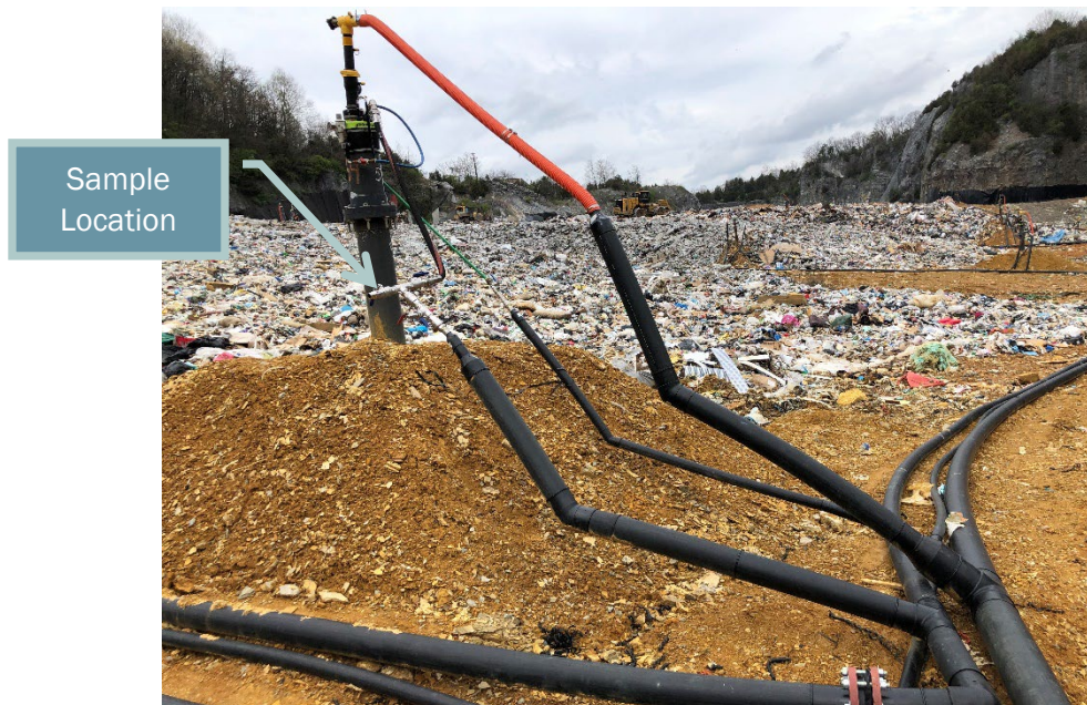
Exhibit 1. Dual-Phase LFG Extraction Wellhead
